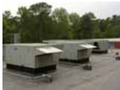
Rooftop AC Units
