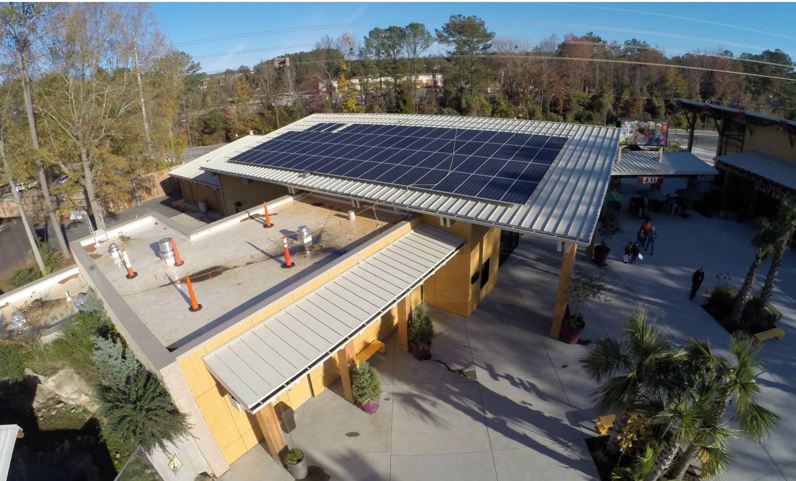
Solar panels atop Riverbanks Zoo and Garden's guest relations center help generate electricity and create awareness about alternative energy.
