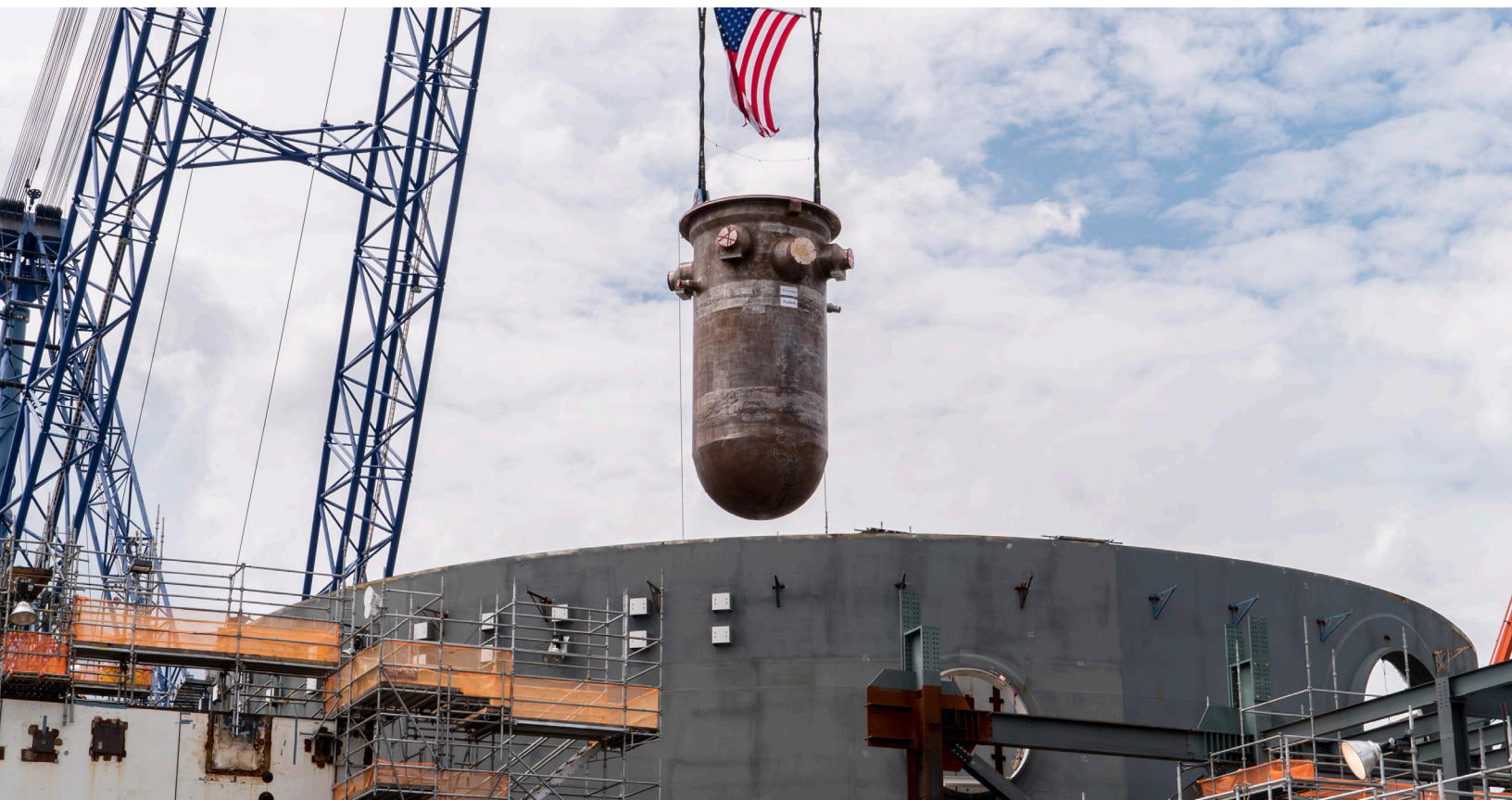
SCE&G and its partners place the reactor vessel in the containment building of V.C. Summer Unit 2.
